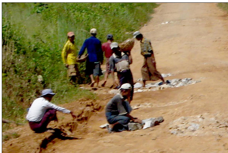
Villages are forced to perform road repairs near Yapu village in November 2008.
